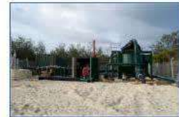
Diesel Powered Pump Station
