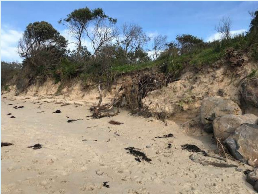
Coastline recession at Flat Rocks - western side of new rock wall at boat ramp, 2 September 2020
