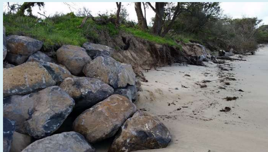
Coastline recession at Flat Rocks – eastern side of new rock wall at boat ramp, 23 August 2020
