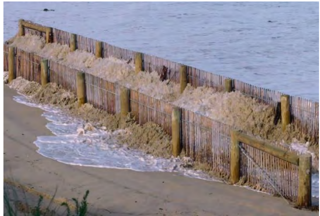
Fig. 39: Double trap sand fence in action, East Beach, Port Fairy (Courtesy: Port Fairy Coastal Group)
