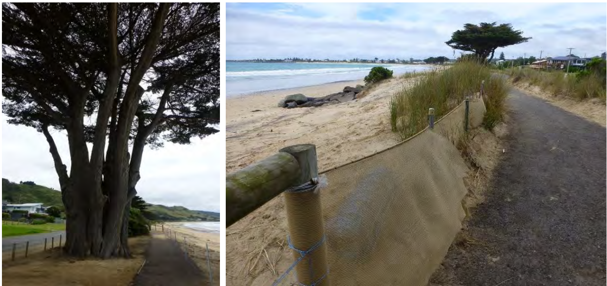
Fig. 47: Dune recession and treatment works, Great Ocean Road, Apollo Bay
