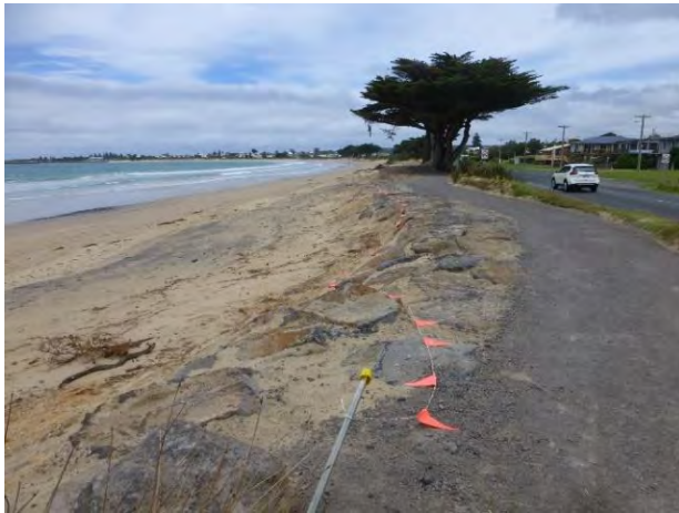
Fig. 48: Erosion adjacent to Great Ocean Road, Apollo Bay
